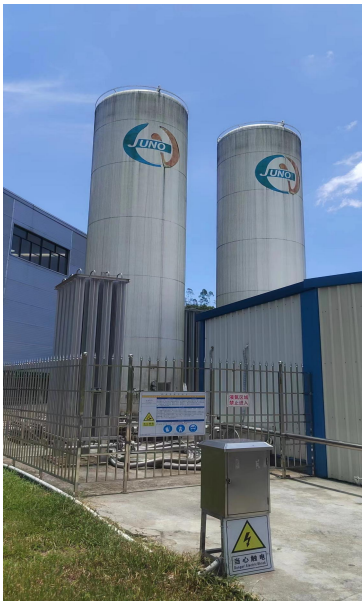
Liquid nitrogen tower
