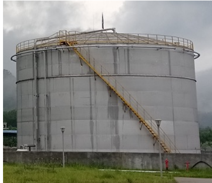
5000 m 3 LAB tank
