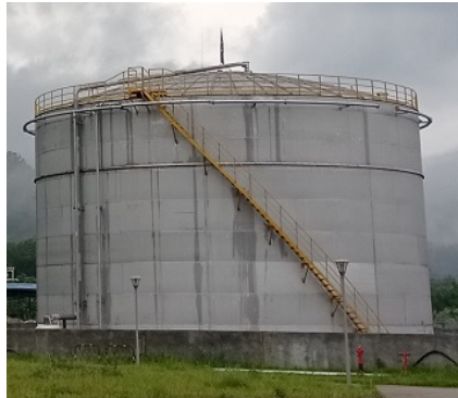
5000 m 3 LAB tank
